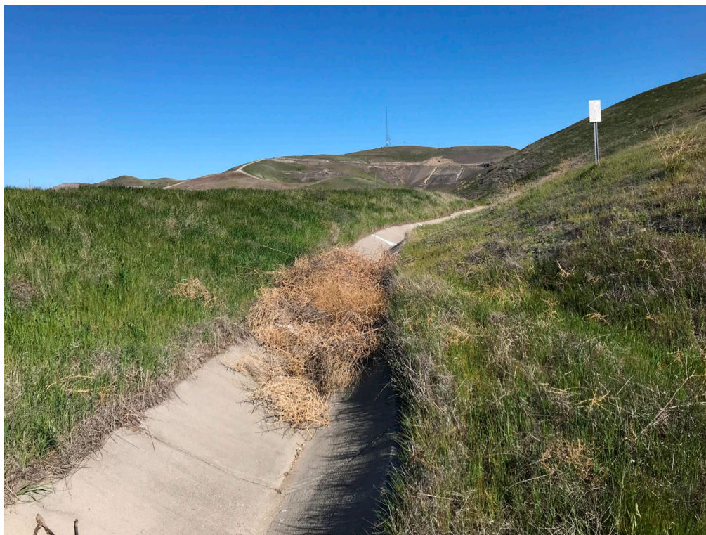
Figure 5 Building 829 Vegetative Debris in Drainage Ditch
