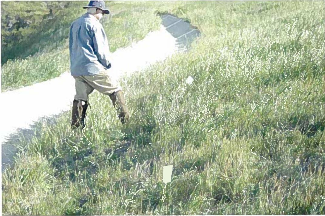
Figure 3 The Length of Crack On the Cap
